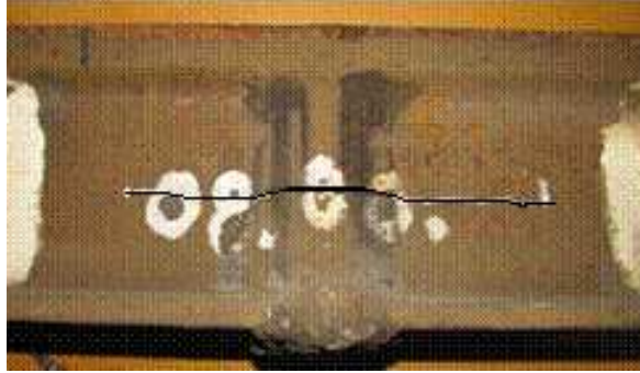
Fig.4. View of a thermic weld score and cracks revealed.
