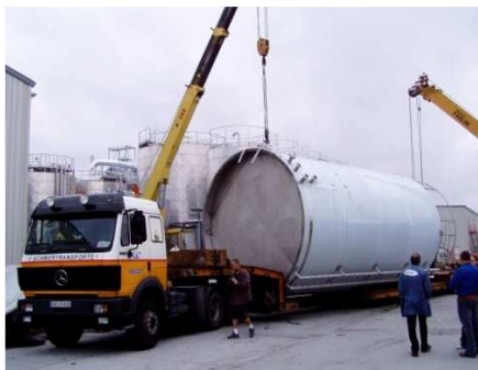
Fig.1. Tank unloading (1100 m 3 )
