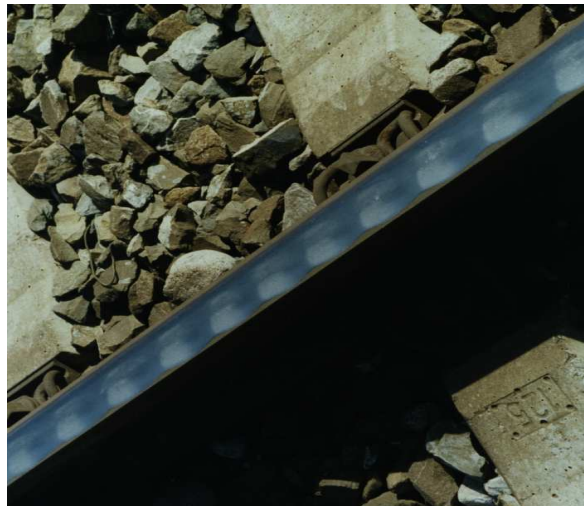
Fig.1. Photograph of corrugations on a rail.
